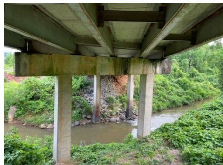
Bridge Piers Show Water Lines From Previous Flooding Events Along Noonday Creek
