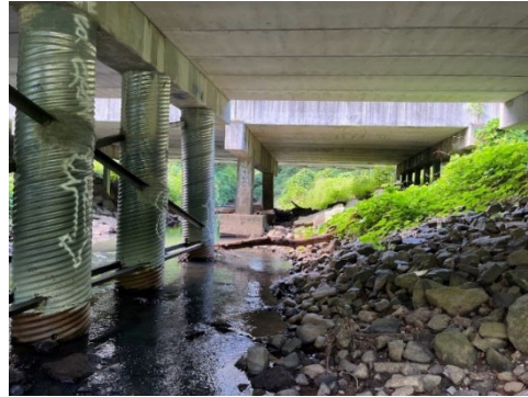
Lower Vertical Clearance And Slope Are Potential Challenges for a Below-Grade Trail Crossing
