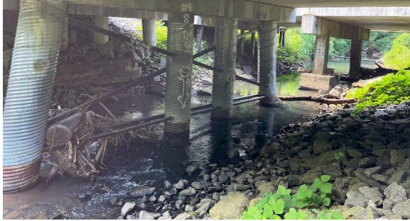
Low Vertical Clearance Beneath the New Chastain Road Bridges
