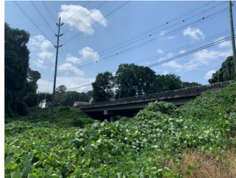
Thick Vegetation Along Utility Easement Looking South Towards Hawkins Store Road Bridge
