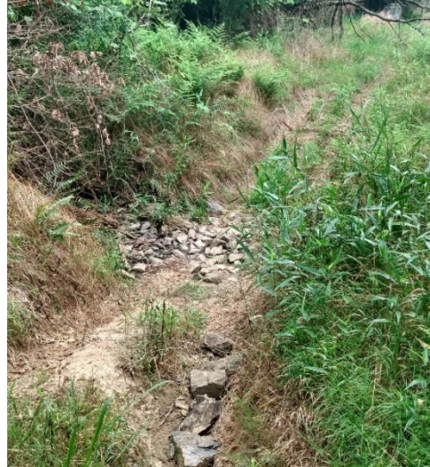
Gravel and Underground Pipes Exposed Within Easement West of the Creek
