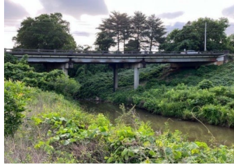
Bells Ferry Road Bridge Over Noonday Creek Looking East from Bells Ferry Trailhead
