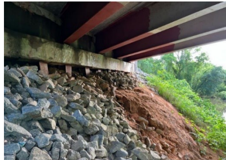
Steep Slopes Underneath the Bells Ferry Road Bridge and Evidence of Erosion
